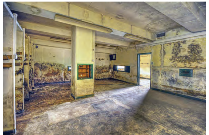
The communication room has been cleared of rubbish and dried out. In the middle of the room a service lift goes up to the AOC office above. Photo Colin Anderson
